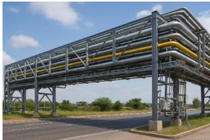
Figure 1. A Typical Industrial Pipe rack in large plant.
