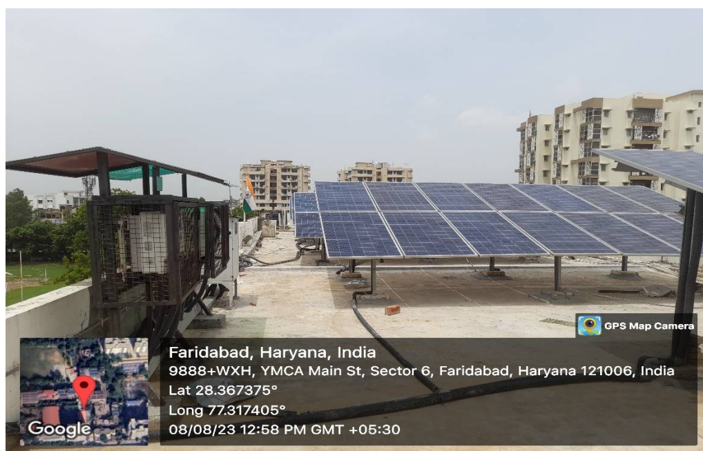
Fig-5.2: Solar rooftop plant
