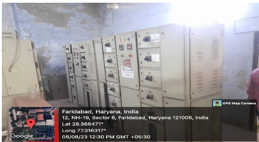
Fig 4.4: 11/0.4 Sub Station Switchgears
