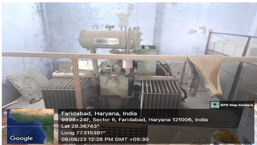
Fig 4.2: 11/0.4 Transformer no 1 (500 KVA)
