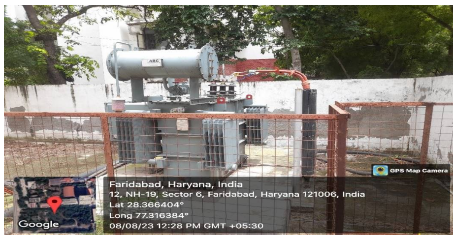
Fig 4.1:11/0.4 Transformer no 2 (1000 KVA)
