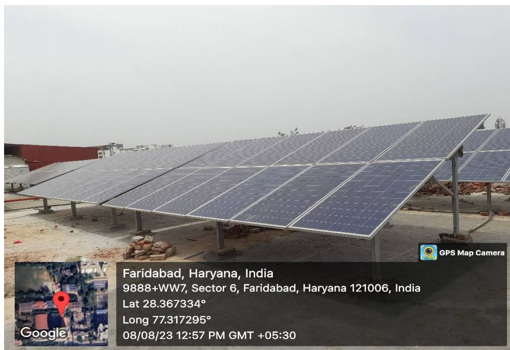
Fig-5.3: Solar rooftop plant
